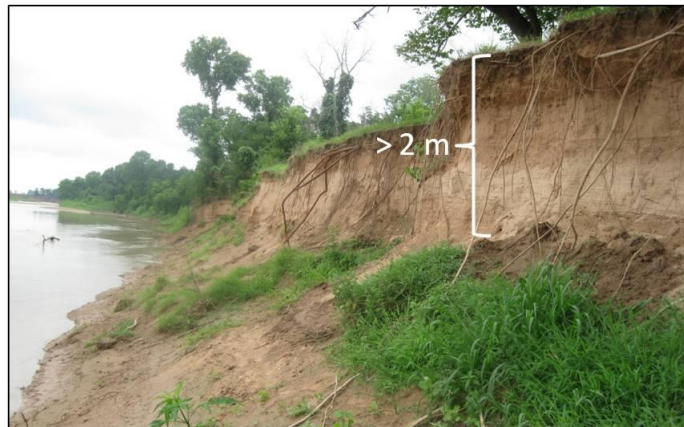
Figure 3.24. Inner bank with slump toe. The vegetation is not extensive along the bank and the area has experienced deforestation since the 1995 time frame. Photography taken by the author on June 30, 2010 at coordinates UTM Zone 14 699413 E & 3453984 N.
