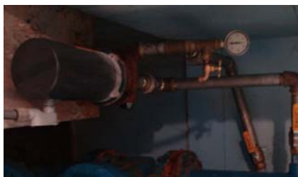
Figure 3.9. Recirculation pump in short term tank 3.
