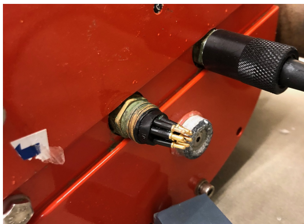
Figure 5.5: Damage to the ADCP bulkhead that was installed at the stern of the turbine deployment platform
