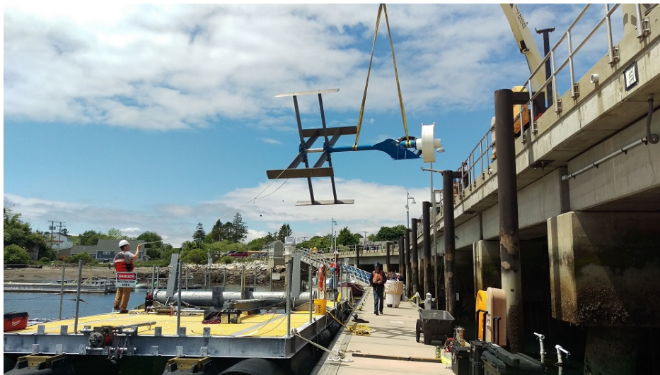
Figure 5.1: Turbine installation in June of 2018 at the UNH Pier in Newcastle, NH
