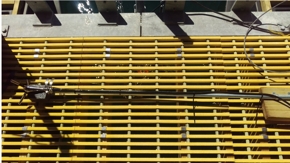
Figure 4.6: Temporary mount used for the first field deployment of an ADV on the turbine deployment platform on 6/15/18
