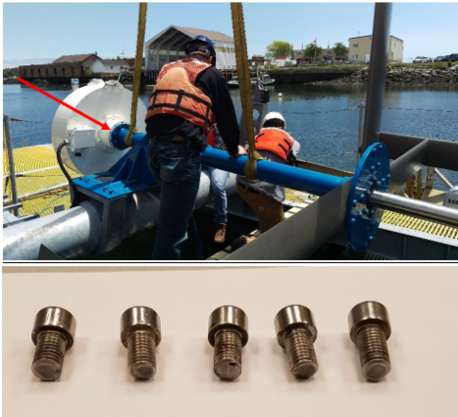
Figure 5.2: Stainless steel bolts sheared in the generator during turbine operation, the location of the bolts is indicated by the arrow in the picture of the turbine
