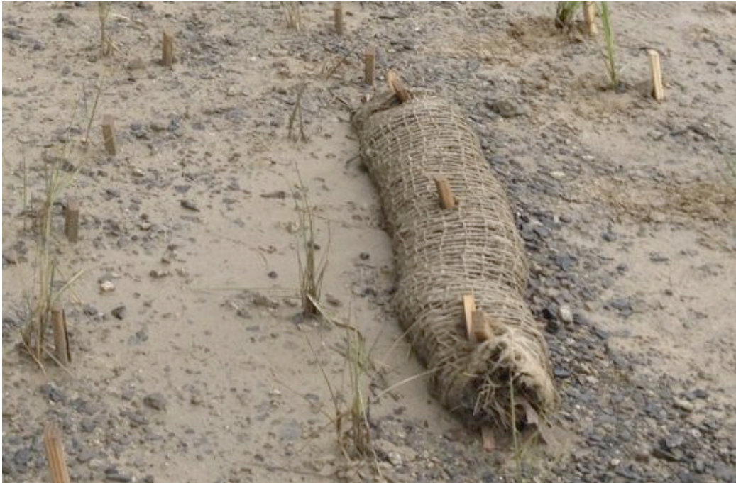
Figure 4. Wave baffle installed to reduce wave energy and erosion. Sand shoreward (left side) and lag deposit of pebbles (right side) of wave baffles.
