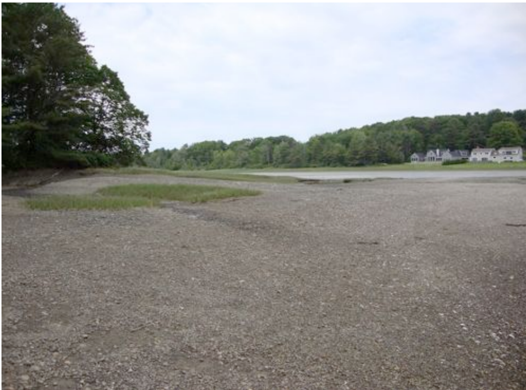
Figure 1. Eroded areas on the southern side of the Wiggley Bridge (top) and the northern side (bottom), before restoration.
