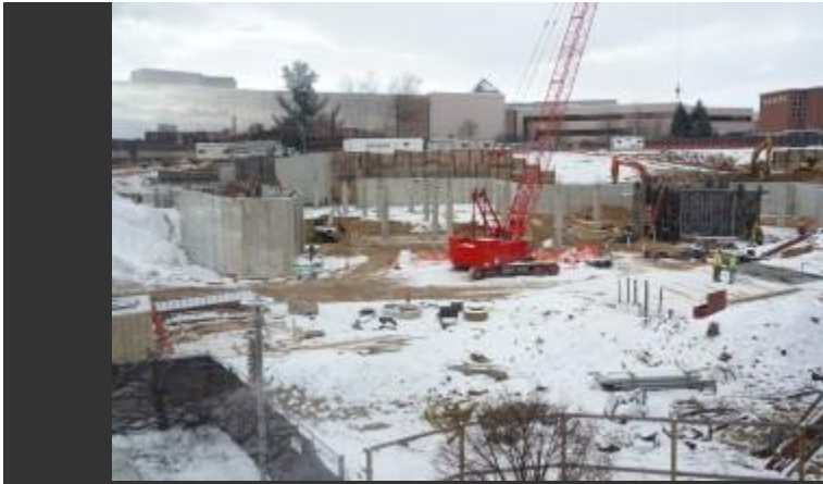
Work is currently underway on the new student center in Hilltop Village.
