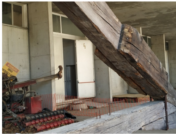
Figure 9 – Example of increased cross-section with timber planks (left) and steel elements (right) [14].
