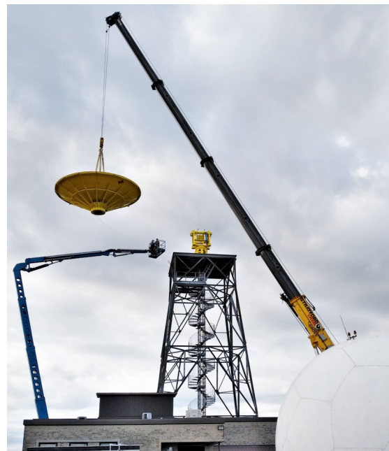
ECCC C-band radar at Exeter, ON being disassembled in order to be put into crates and moved to a Western Engineering facility.
