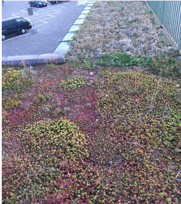
Plate 7.1 A green roof in Copenhagen, Denmark (Rumble, 2012). Sedum spp. in the foreground are coloured red, indicative of drought stress (Teeri et al. , 1986). The difference in plant morphology seen in the mid-ground corresponds with a change in substrate depth, with the section furthest away shallower in depth.
