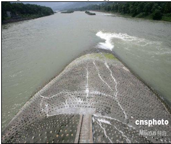
Image 1: Cracks in Dujiangyan dam
