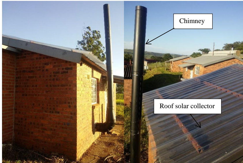
Figure 4.1 Picture (a) on the left shows the modified storage and picture (b) on the right shows the solar collector system for heating incoming air.
