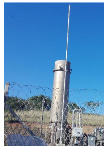
Figure 2d: Methane gas extraction flare
