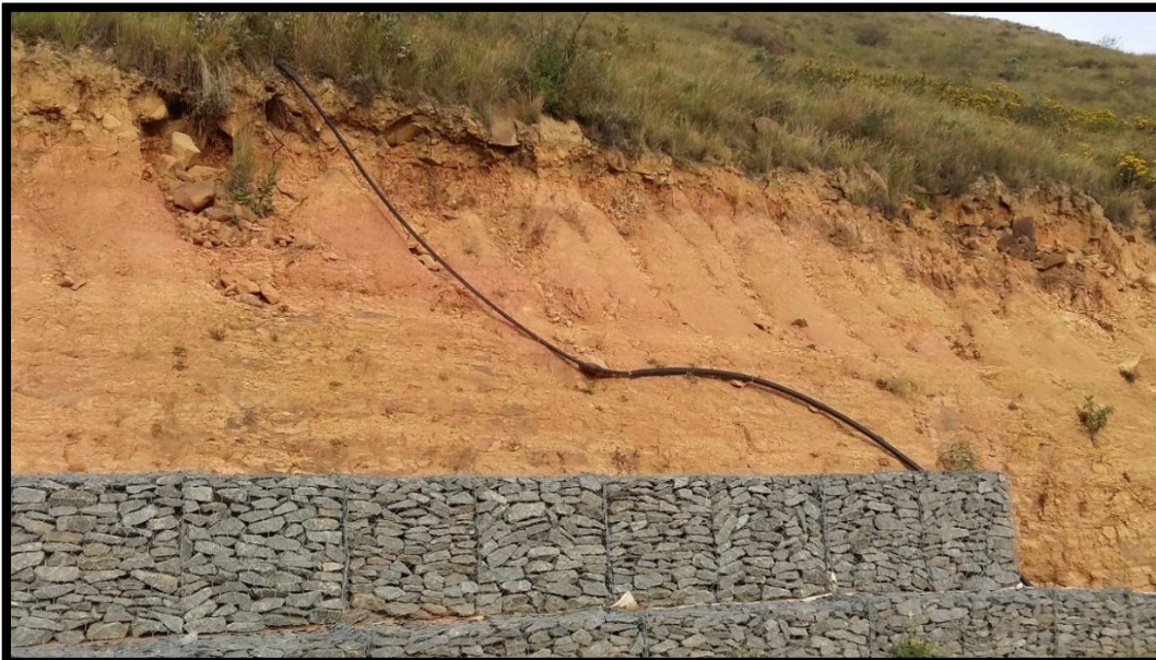
Plate 5.3: Water Connection Pipes Feeding off to Residents in Ward 2
