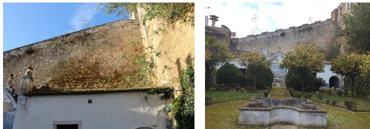
Figure 4 – Wall section at the north of Independence Palace garden: (a) general view and (b) detail of the wall
