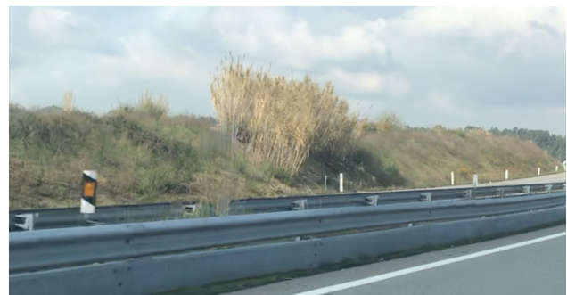
Figure 13. Arundo donax growing on one of the slopes of the A29 highway, in the Estarreja region (central area of Portugal)
