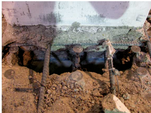
Fig. 9—East side of connection region in Specimen B2 after severely degraded concrete had been removed by hand.
