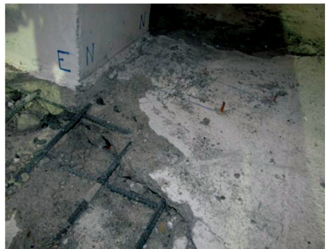
Fig. 8—Damage in slab north of column in Specimen B1.
