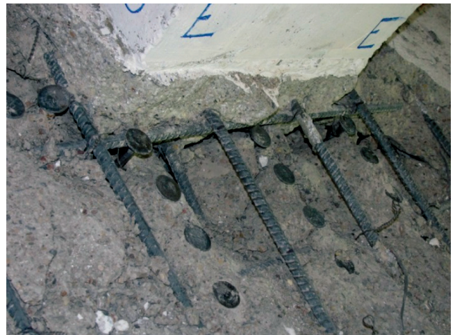
Fig. 7—Void in connection region, typical of damage at east, west, and south column faces of Specimen B1.
