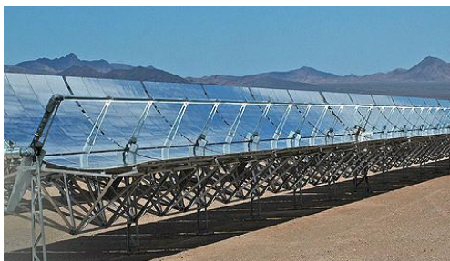
Figure 6. A PTC-based solar thermal power plant in the U.S. [9].
