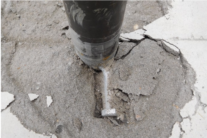
Figure 11. Concrete failure of stud connectors.
