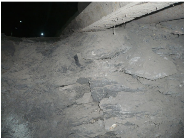
Figure 4. General view of floor rocks shear of a belt roadway of western longwall 12 of seam c_{18}
