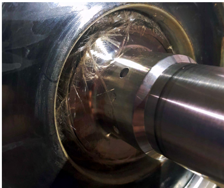
Figure 11: Photograph of the damaged turbo-generator with unwound glass fiber between rotor and stator.
