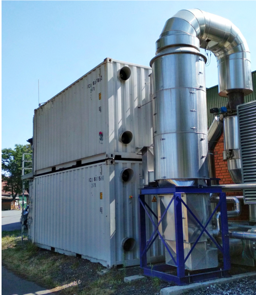
Figure 5: CORC plant in modular design with the direct evaporator and HE 1 in the front, connected to the setup in the containers.
