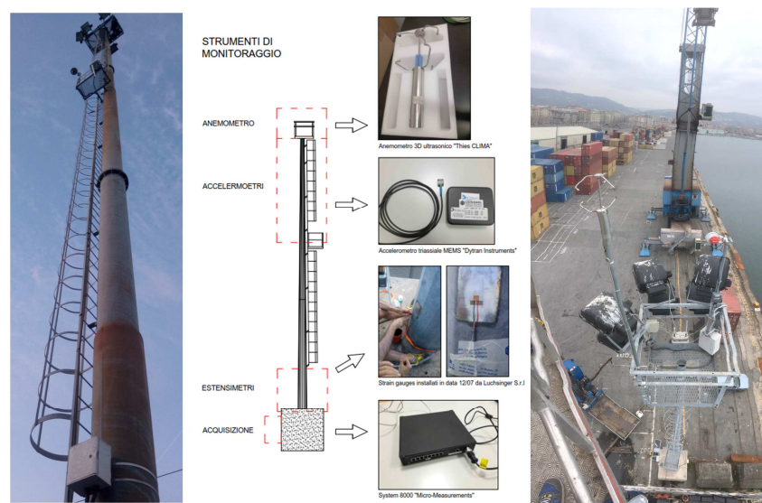
Figure 14 - Full-scale monitoring of a steel tower in the Port of La Spezia
