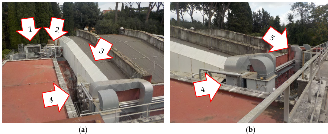
Figure 3. Top view of Aula Magna. (a) Left side; (b) Right side. (1) Heat Pump; (2) Pumps and storage tanks; (3) Duct protection carter; (4) and (5) Air Handling Units.
