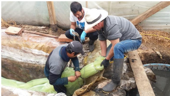
Program participant helping to install a biodigester at a farm in Sesquilé, Cundinamarca. Photo: Fomento Ganadero-Alquería.
