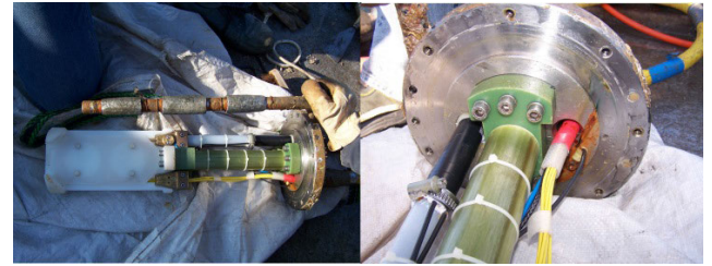
FIGURE 12. Pictures shows the interior of the Underwater termination box with rust showing the water level.
