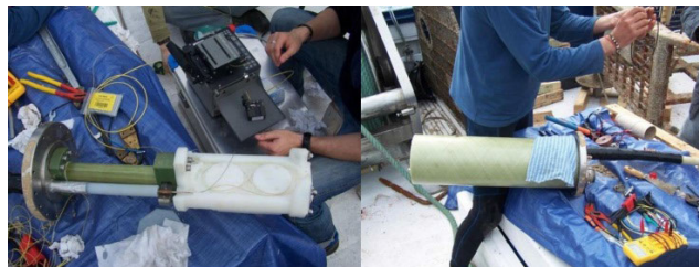
FIGURE 14. Termination box and the optical fiber connection.
