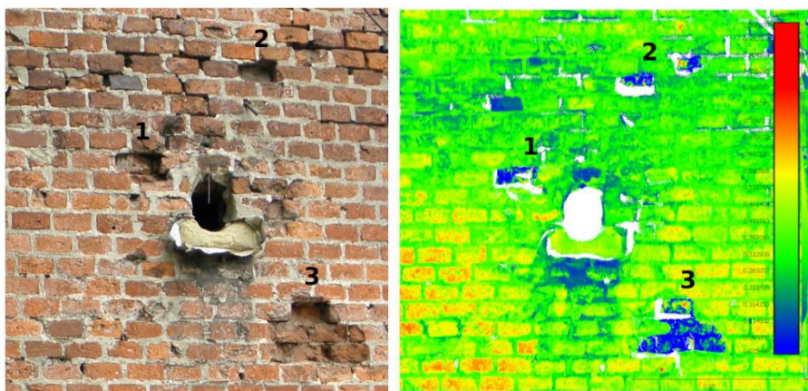
Figure 5. Presentation of cavities in the RGB picture and on the point cloud
