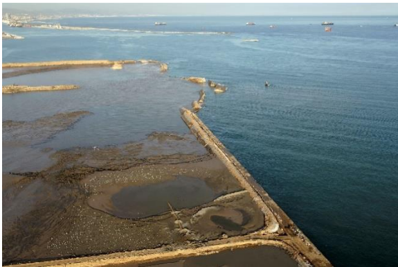
Figure 32. View of the Prat quay failed section
