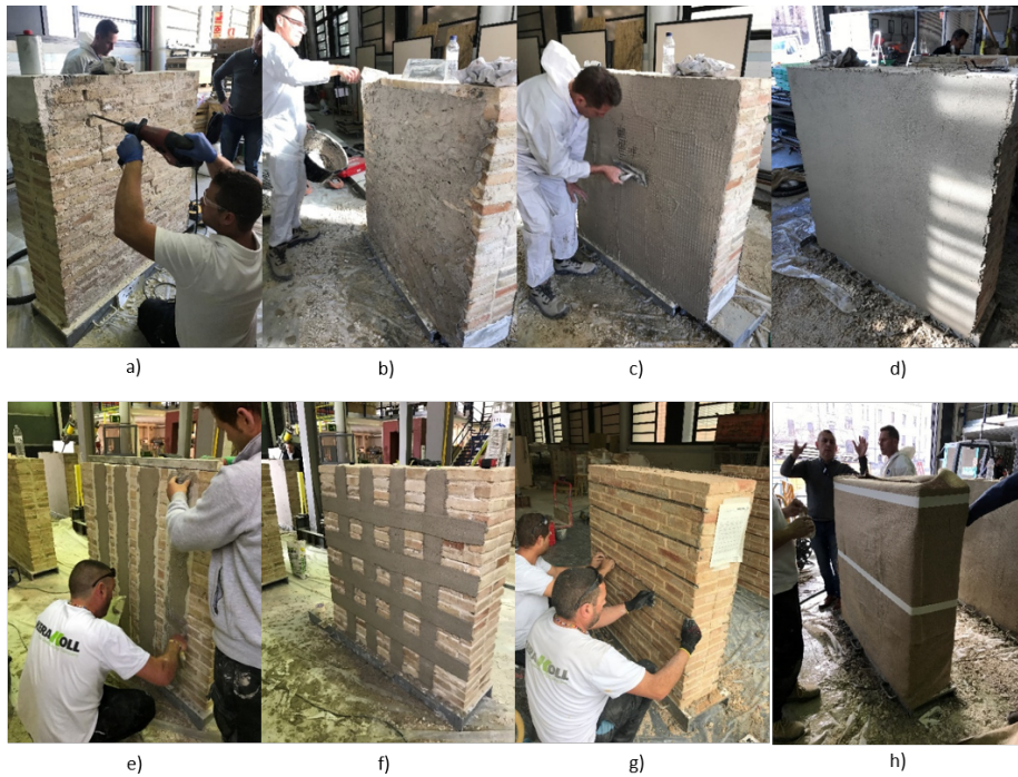
Figure 1: Procedure for the application of the TRM systems: a) creation of grooves along the mortar joints, b) application of the first layer of mortar, c) set of the fibre net, d) finished look of the wall retrofitted with basalt TRM, e) application of the first layer of vertical mortar strips, f) finished look of the wall retrofitted with steel TRM, g) insertion of the helical stainless steel rebar, h) wrapping of the specimens with wet sackcloth fabric for curing
