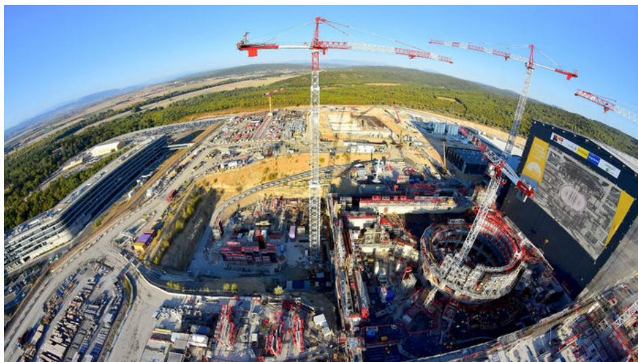
Fig. 1.5. Construction site of ITER project, late 2017 [Credits: ITER Organization online site www.iter.org ]
