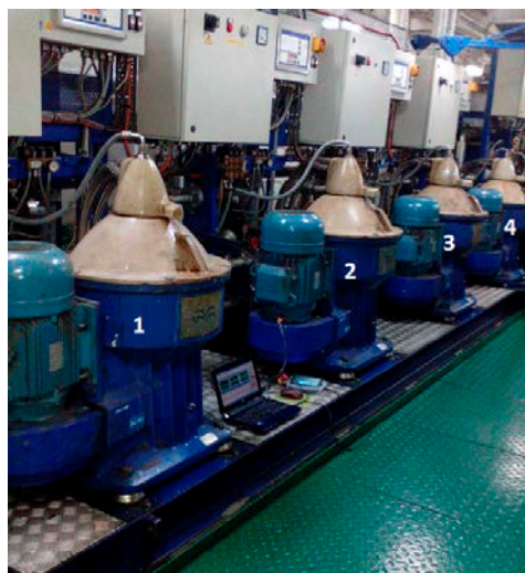
Figure 1. Photography of four marine oil Separators Alfa Laval SA 831 labeled with their corresponding numbers.
