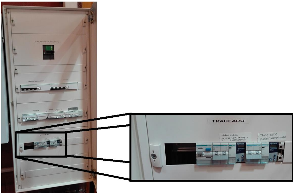
Figure 54: Heat Tracing switches.
