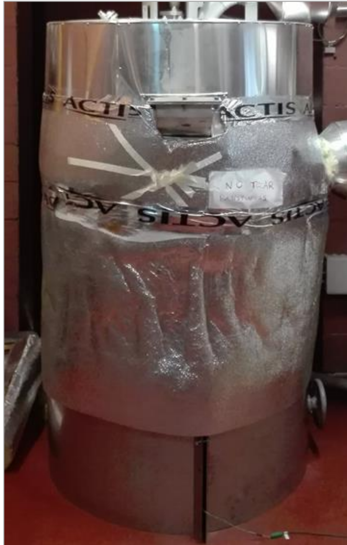
Figure 18: Storage Tank where the molten salts are melted.
