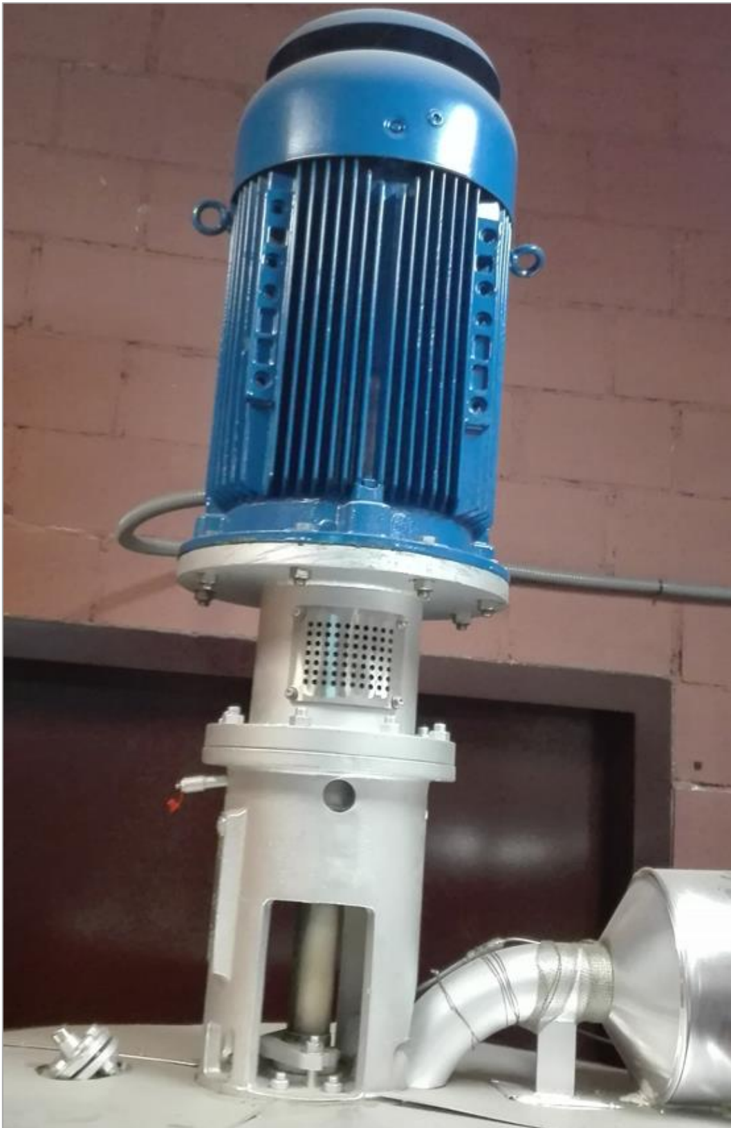
Figure 20: Visible section of the pump.
