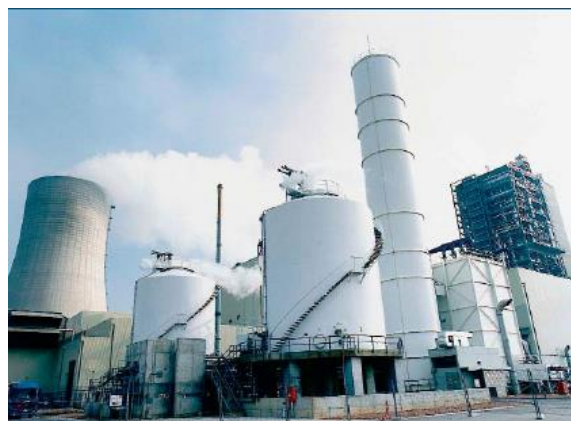
Figure 28. From left to right; refrigeration tower, storage units, distillation tower and heat exchangers [3].
