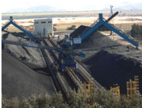
Figure 24. ELCOGAS power plant's coal storage yard [3].
