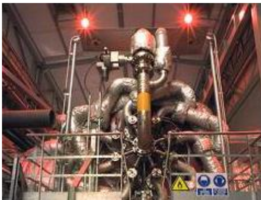
Figure 27. GT operating position [3].
