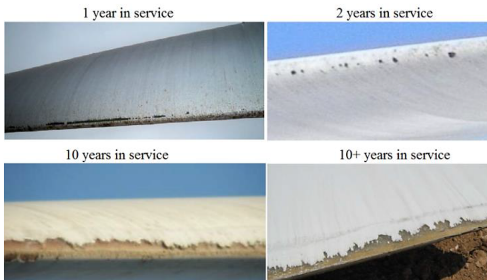
Figure 27: Blade erosion progression in field use [16].
