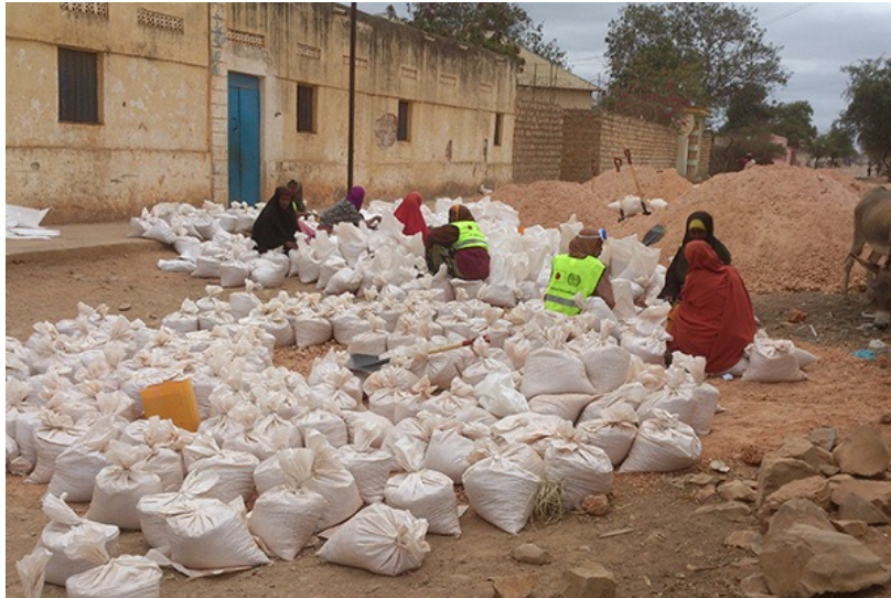
Photo 1: Female villagers preparing Do-nou by filling gunny bags with murram (a clayey material used for road building) ( http://corekenya.org/gallery/ )
