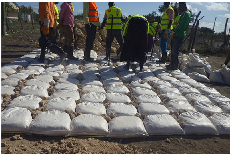
Photo 2: Do-nou's are lined up after being flattened ( http://corekenya.org/gallery/ ) to underpin an all-weather road
