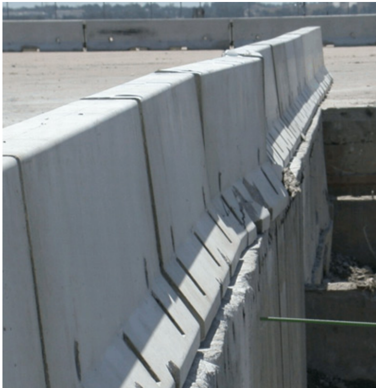
Figure 25. System Damage, Test KTB-1
