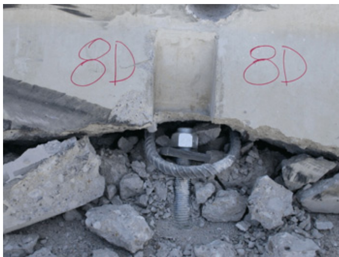
Figure 28. Barrier No. 8 Tie-Down Anchor Damage, Test KTB-1
