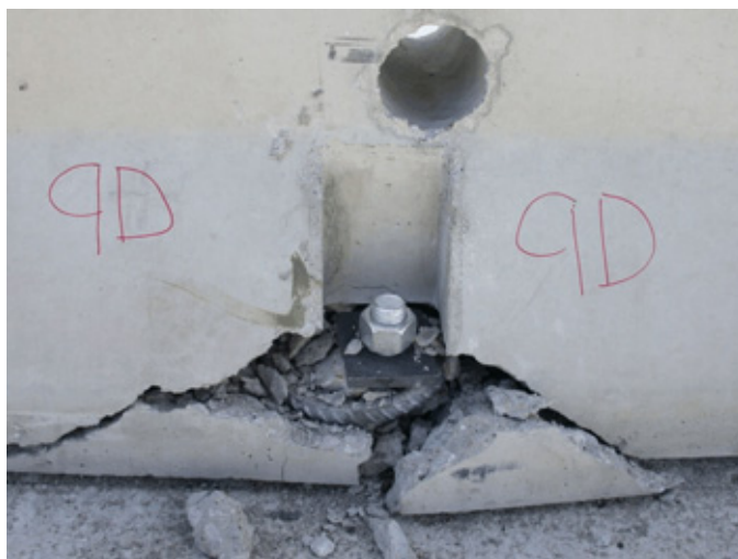
Figure 29. Barrier No. 9 Tie-Down Anchor Damage, Test KTB-1
