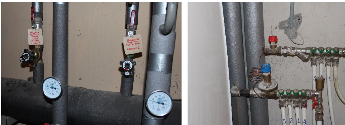
Figure 11 - Balancing valves for HVAC systems
