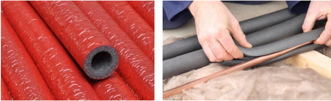
Figure 9 - Pipe insulation and insulated distribution pipes of HVAC systems
