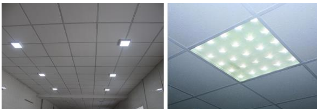
Figure 15 - LED lighting fixtures
