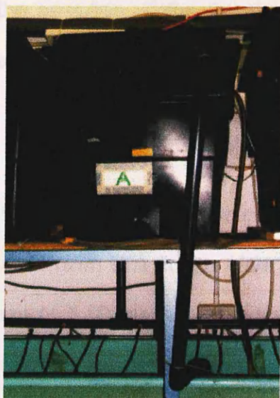
Plate 14. Header tank and water distribution line.
