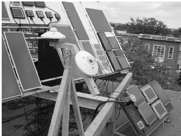
Figure 2.1: Rooftop elements of the CREST outdoor measurement system
