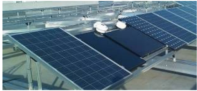
Figure 5 Dedicated reference modules and irradiance sensors installed at Gent.
