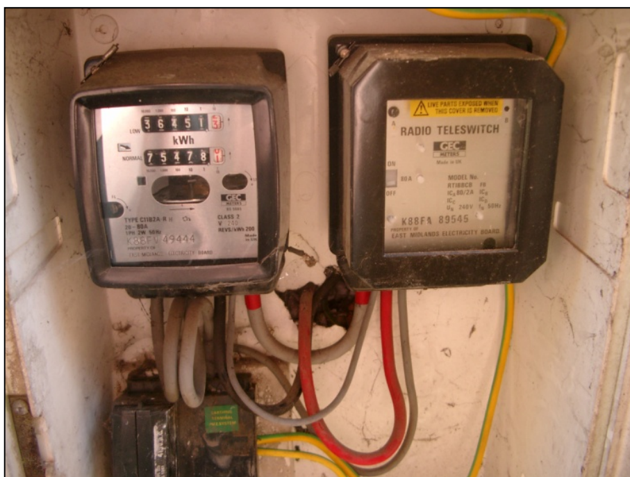
Fig. 58. Domestic Meter Cupboard
