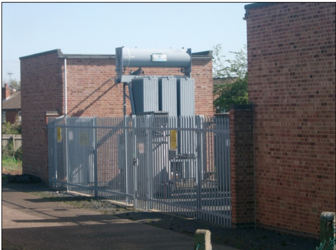
Fig. 54. 33 /11 kV Primary Substation, East Midlands, UK
