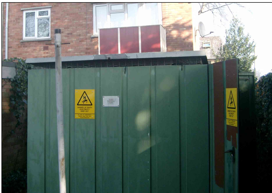
Fig. 56. 11 kV / 400 V Enclosure mounted secondary substation
