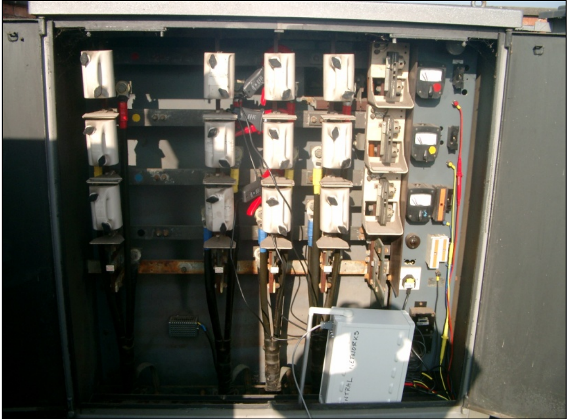
Fig. 57. Low voltage circuit distribution board
