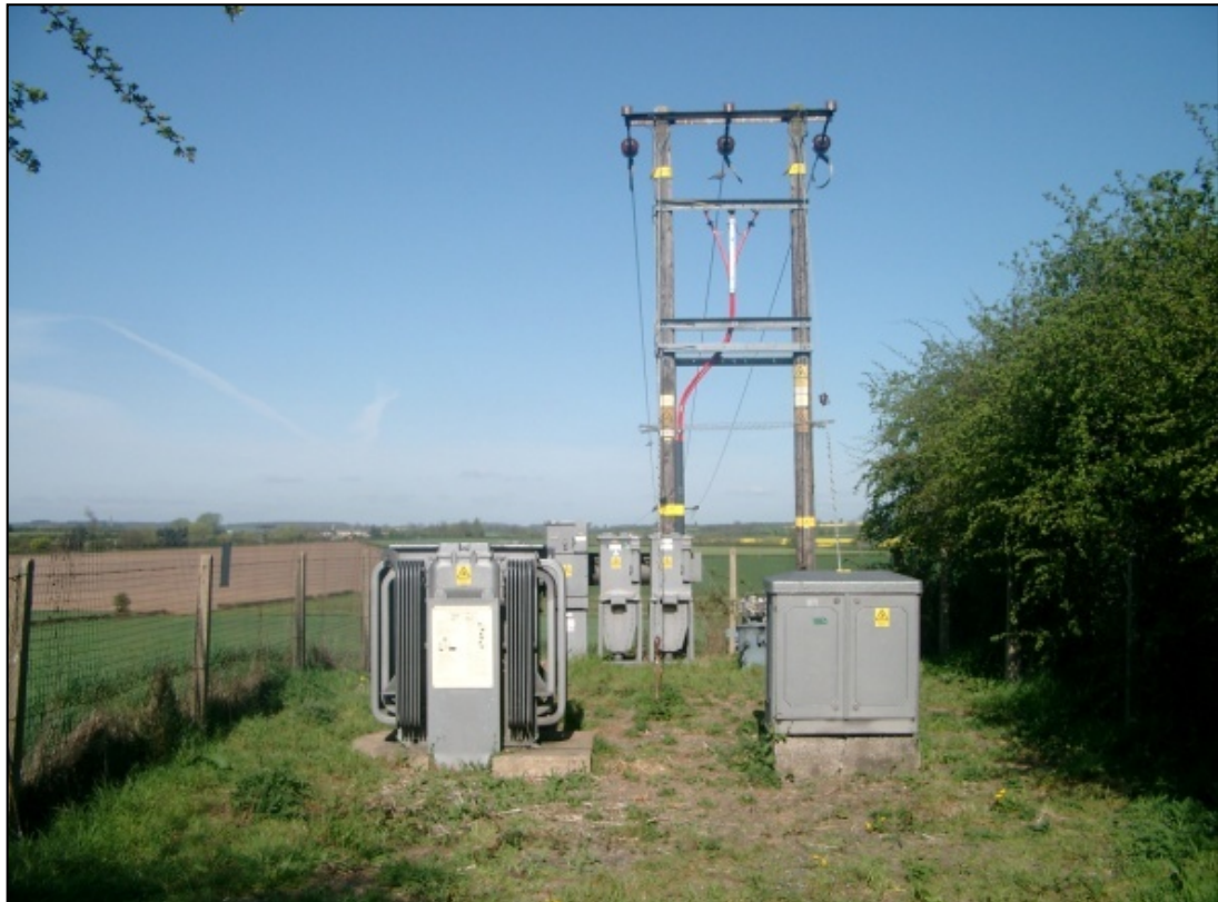
Fig. 55. 11 kV /400 V Secondary substation, East Midlands, UK
