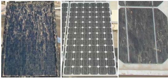
Figure 2: Accumulated dust on different PV modules installed in Kuwait.
