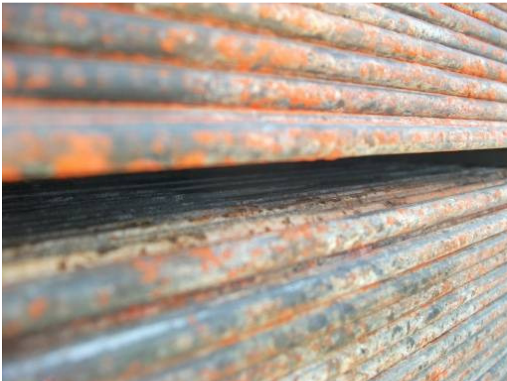
Figure 5: Corrosion condition of a section of the Humber Bridge main cable
