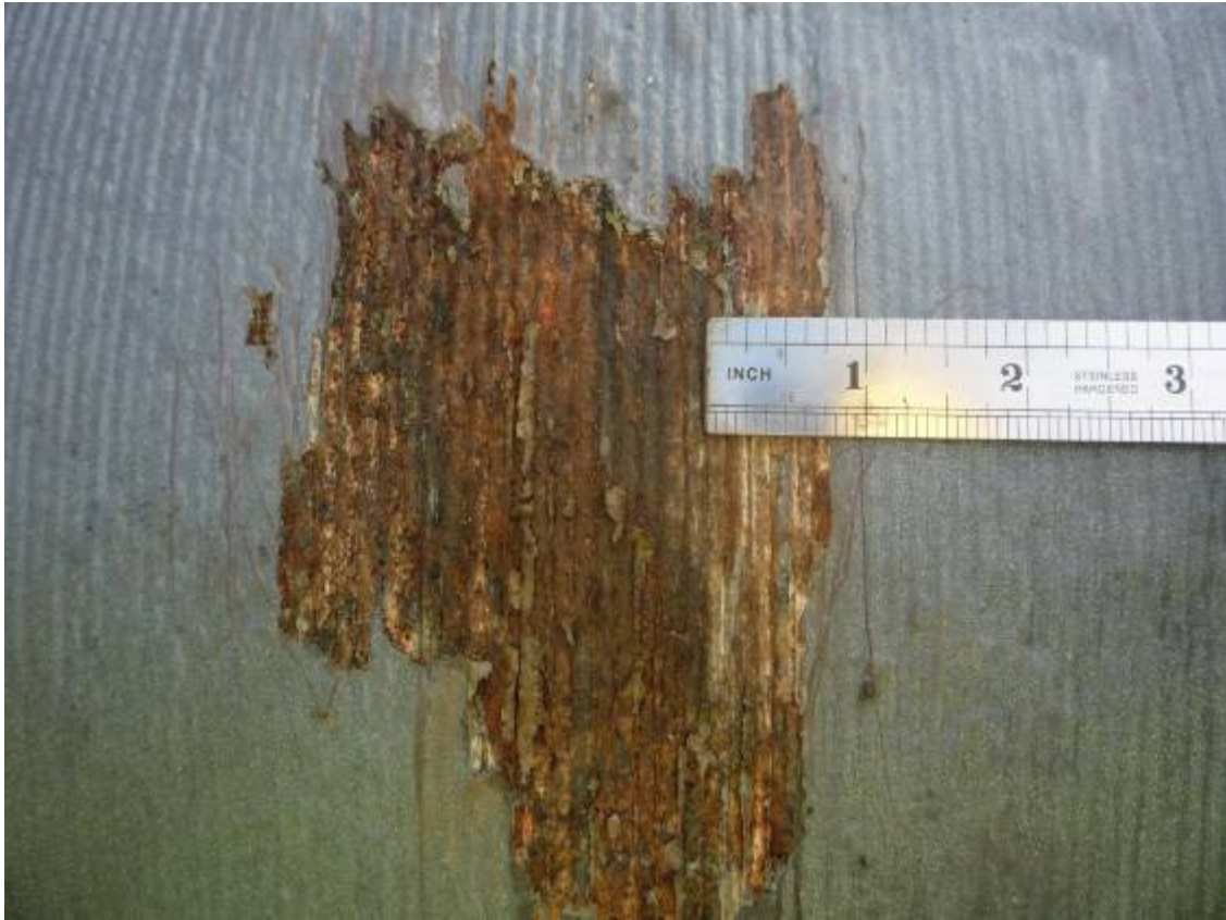
Figure 9: Typical outer skin corrosion damage
