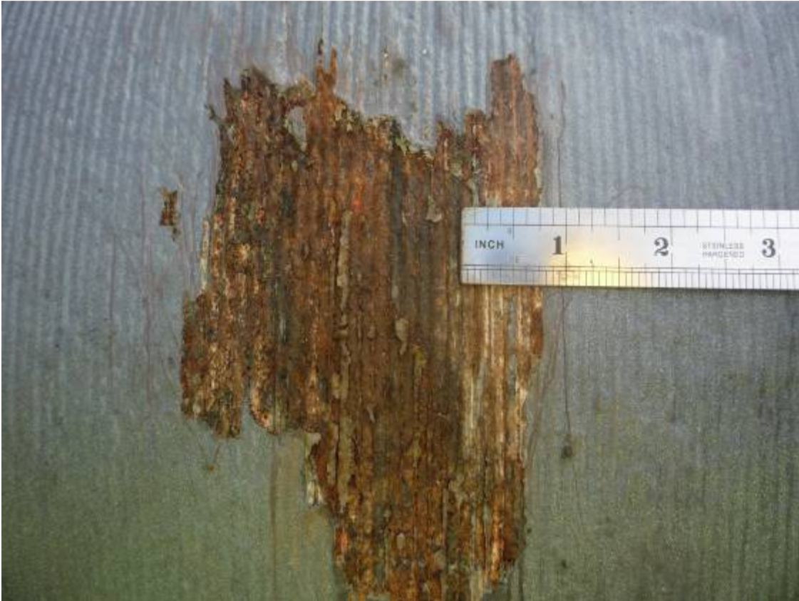
Figure 9: Typical outer skin corrosion damage
