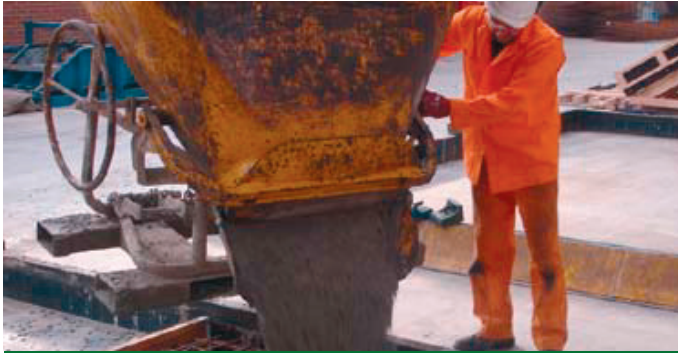
SCC being used in the production of stairs and landings at Hanson Building Products, Hoveringham.
