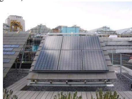
Figure 4 Picture of a 1kWp high-efficiency system on a roof top in London.
