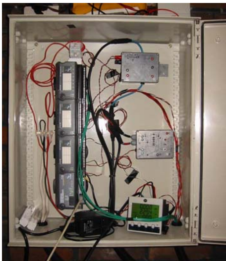
Figure 5 Picture of the monitoring system. The FP-2000 data logger (left) records DC current from a current transducer box (top right) and DC voltage from a voltage divider box (middle right). AC current and voltage are recorded from the output of a ND Multi Cube multimeter (bottom right).
