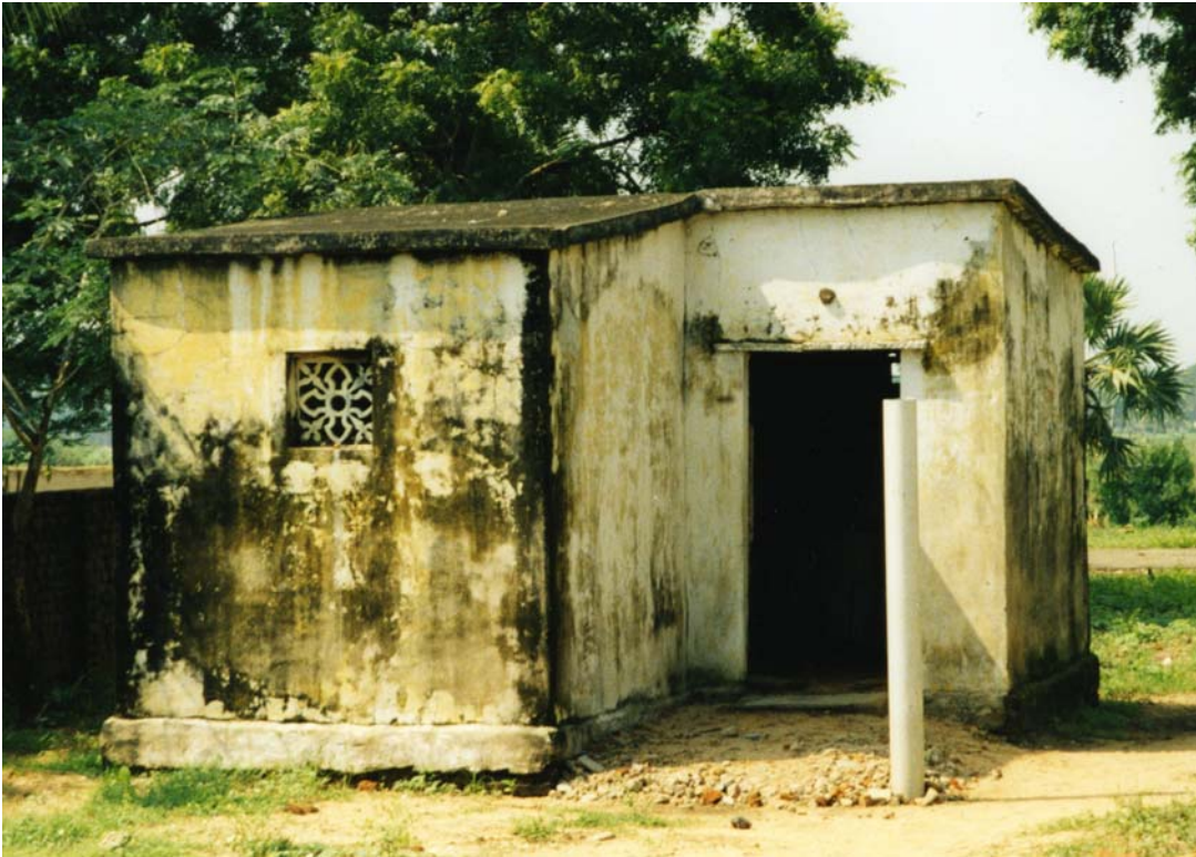
Figure 3: Example of a ‘cyclone resistant house’ built in 1998 (East Godavari, Andhra Pradesh). (Source: Author)
