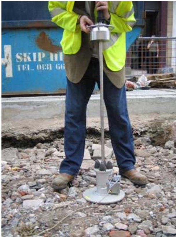
Figure 1. Lightweight Deflectometer – in use on compacted recycled crushed demolition rubble. Note the 300mm diameter plate, the falling mass ready for release from a high drop height, and the four rubber buffers which damp the impact and control the load pulse duration. This model is shown with a hardwire transmitting the load cell and geophone measurements.
