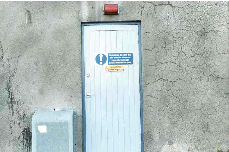
Figure 9. Cracking due to inadequate curing (photograph)
