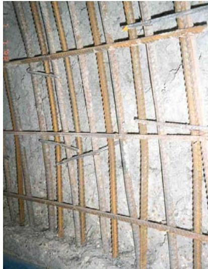
Figure 4. Brick archway strengthening at Lancaster Place Vaults (before application of sprayed concrete) (photograph)
