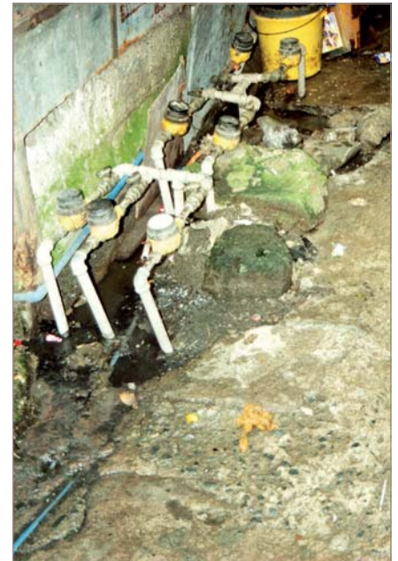
Fig. 2. In poor parts of Manila, the water concessionaire has installed banks of water meters to which households can legally connect their own supply pipes
