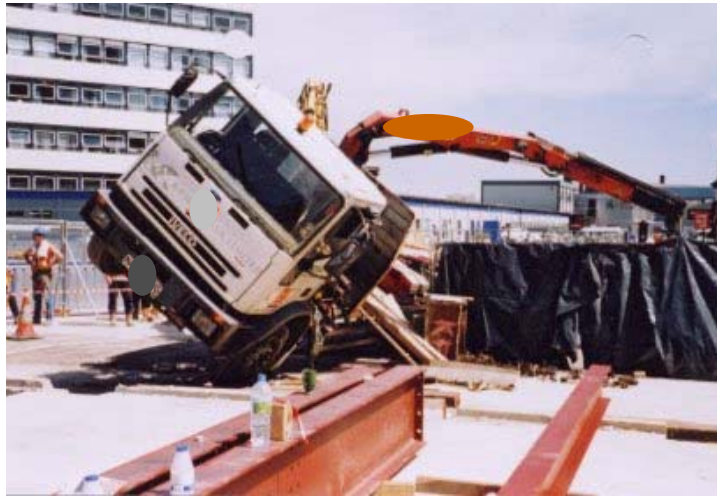
Figure 5 Dangerous occurrence involving access and space constraints (11)
