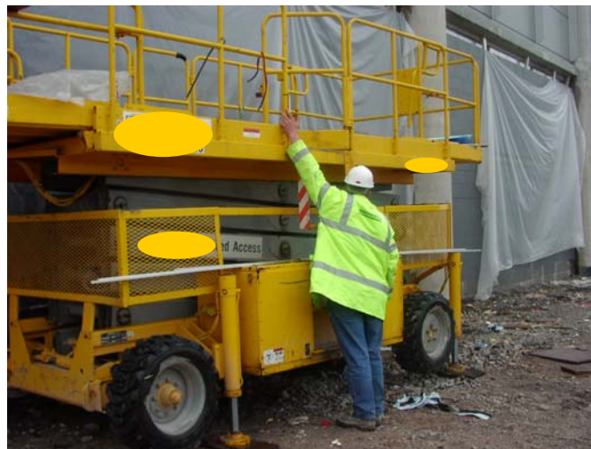
Figure 7 Poor foot and handhold provision on scissor lift (6)
