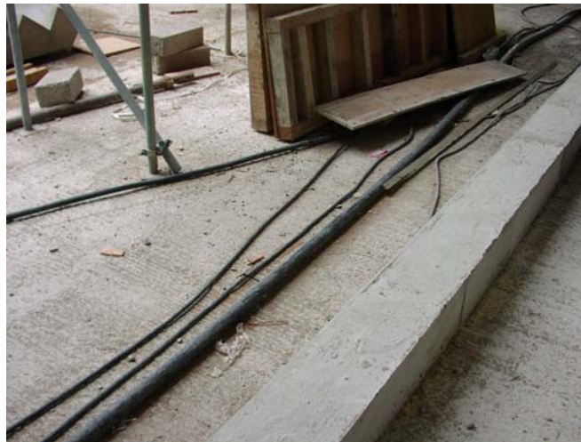
Figure 6 Presence of trip hazards (17)
