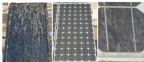
Figure 1: Accumulated dust on different PV modules installed in Kuwait.
