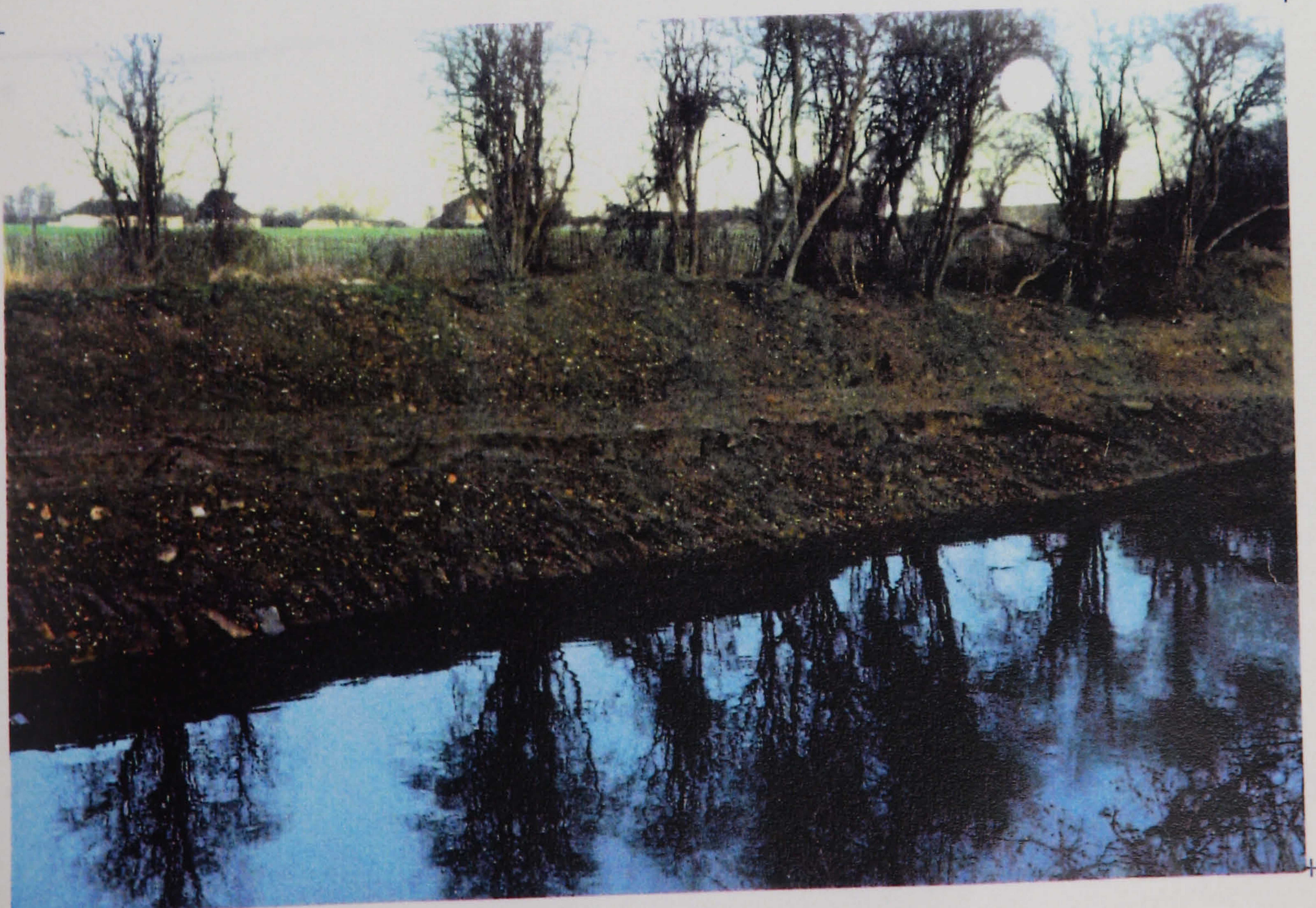
Figure 8.16 Iver - location of tension cracks
