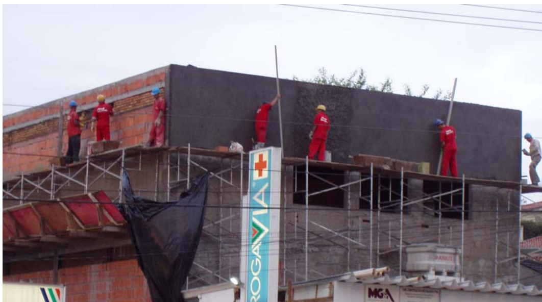
Figure 8 Helmets worn but handrail missing
