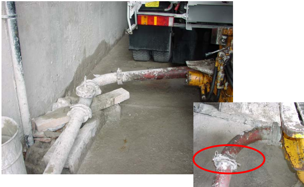
Figure 7 Concrete pump connection problems
